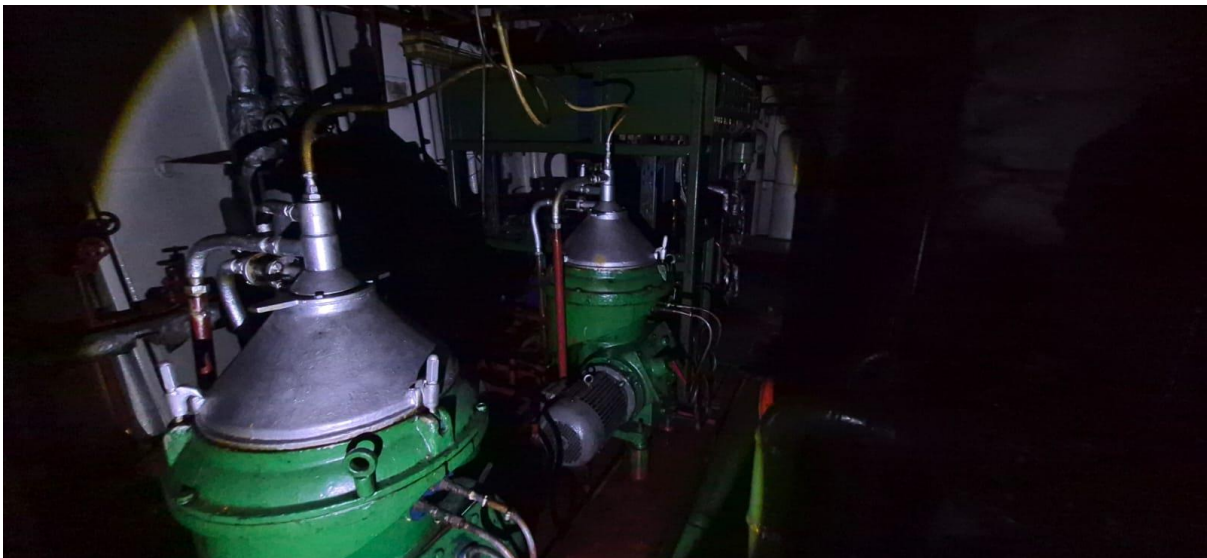
Image 31: 2x Heavy Fuel Oil Purifiers
