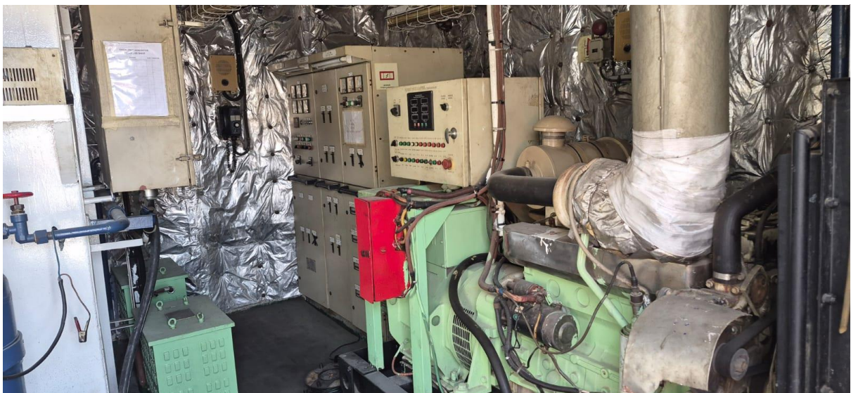
Image 27: 60 kW Emergency Generator Room
