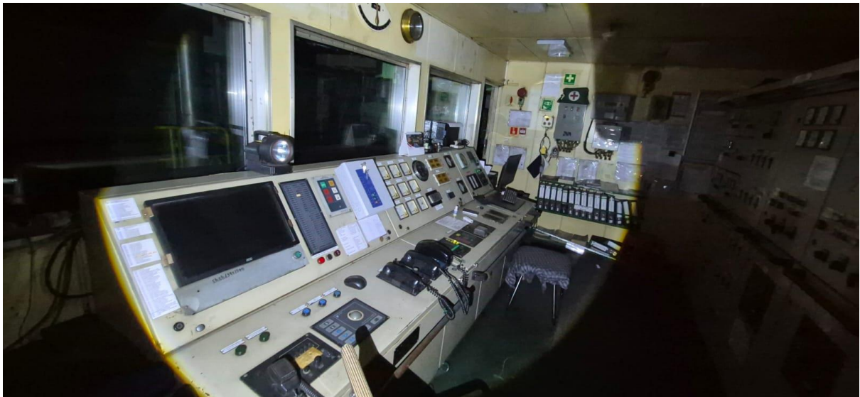
Image 20: Main Engine Control Room
