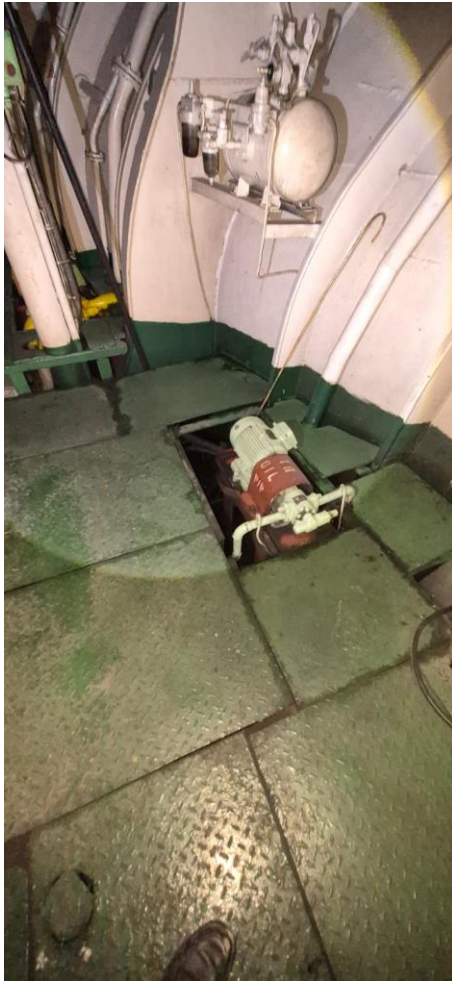
Image 28: Diesel Oil Transfer Pump
