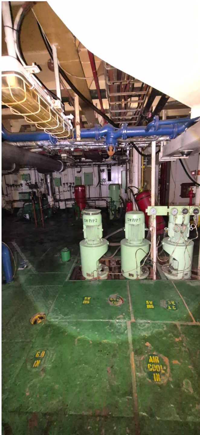
Image 23: Main Engine Sea Water Cooling Pumps
