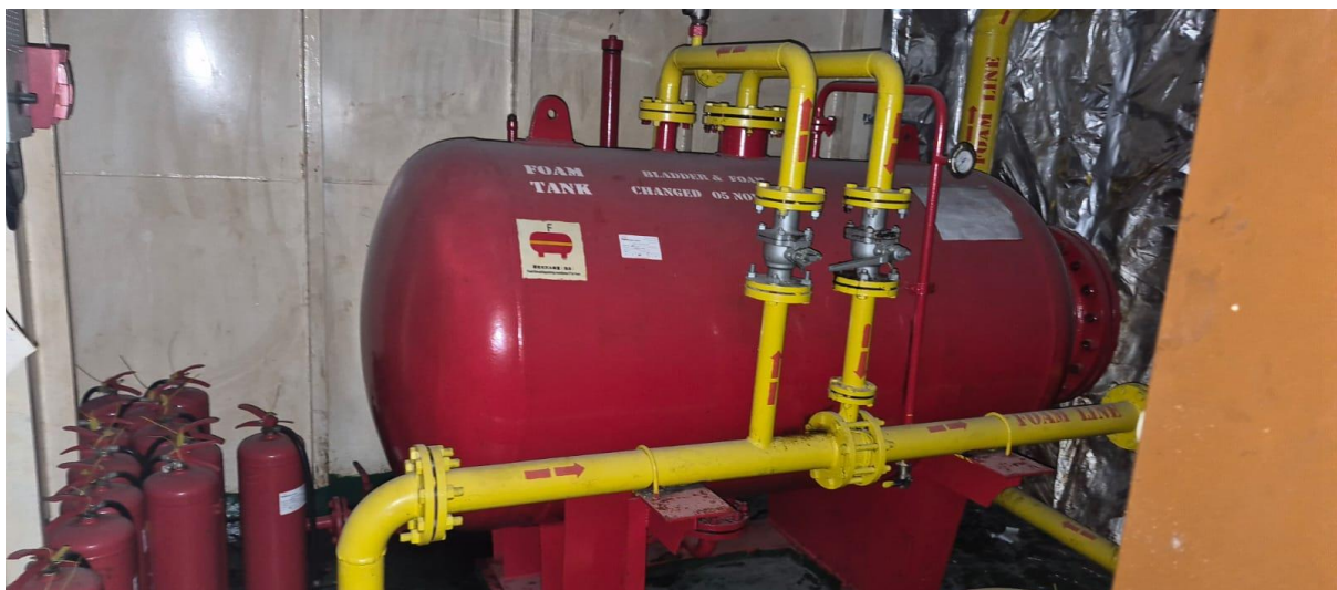
Image 38: Fire Extinguishing Foam Tank
