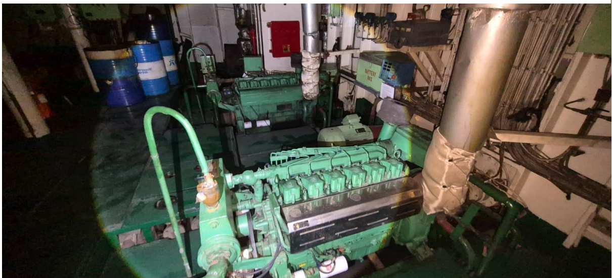
Image 26: 2X250 kW Main Generator
