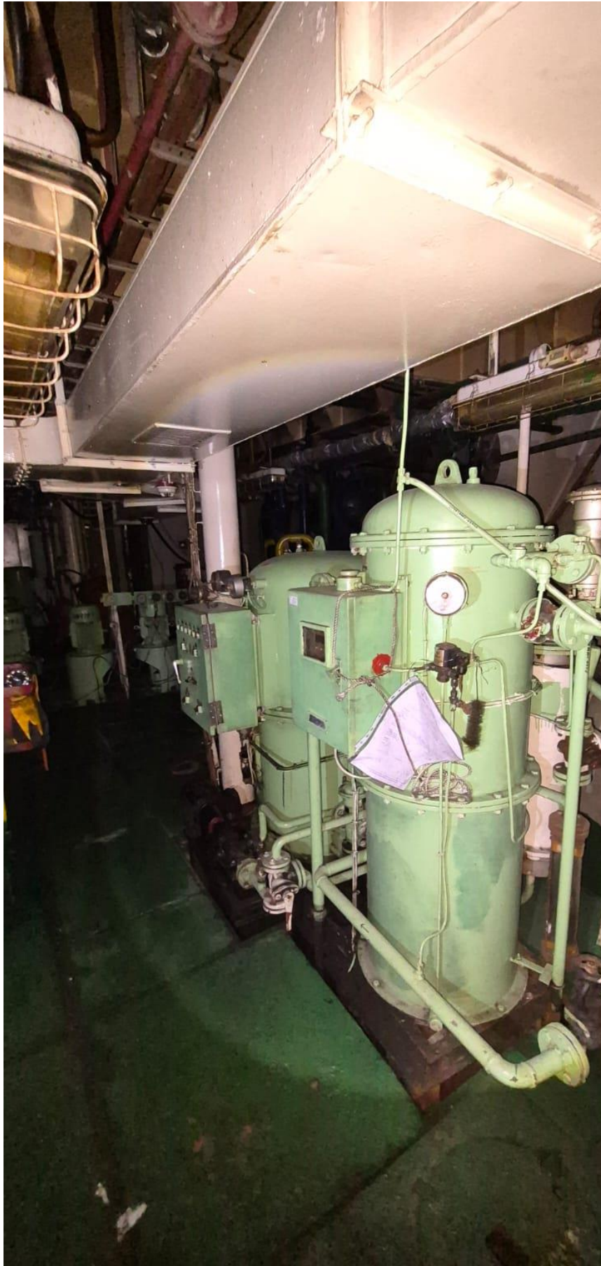
Image 35: Bilge Oily Water Separator
