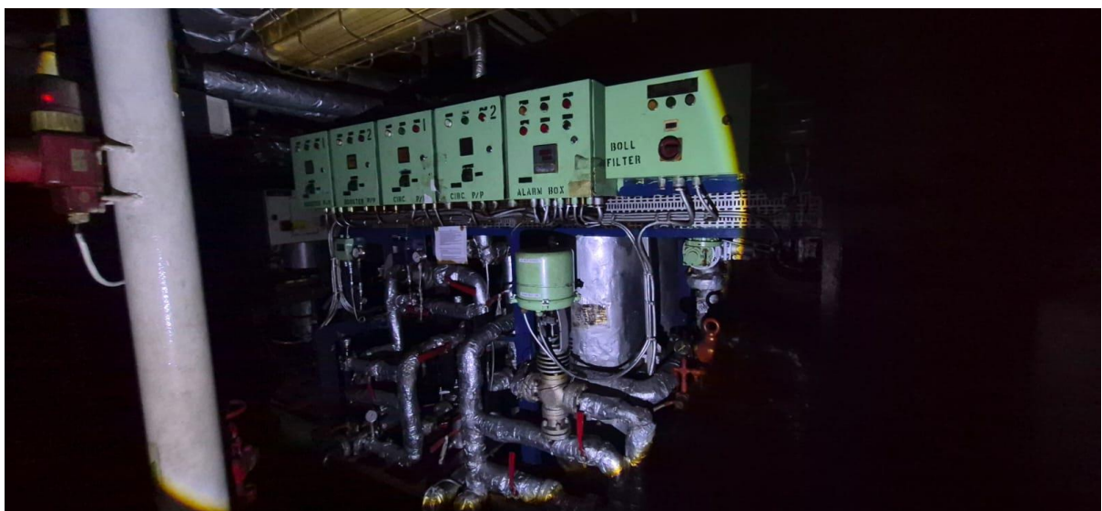
Image 34: M.E. Heavy Fuel Oil Pumps
